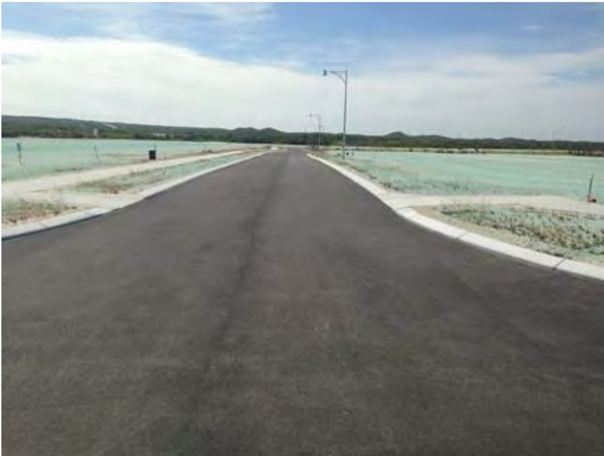
First stage completed internal roads and lots. Note all internal power, water and waste water infrastructure has been installed.
