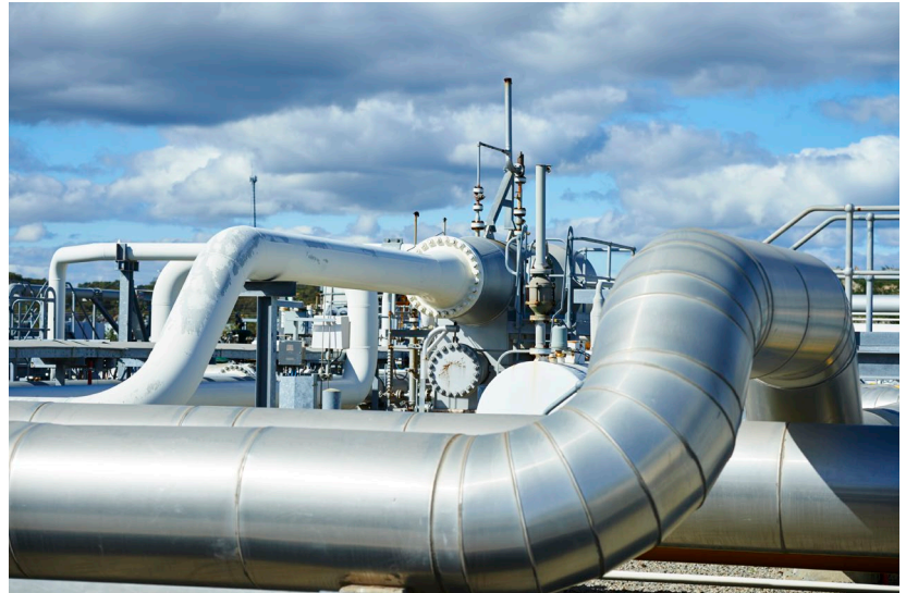
Figure 9.7: Compressor Station 10 in Kwinana
