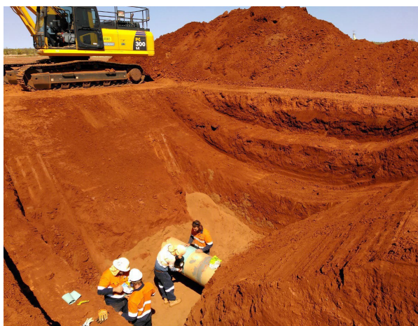
Figure 1.2: DCVG and example of corrosion
