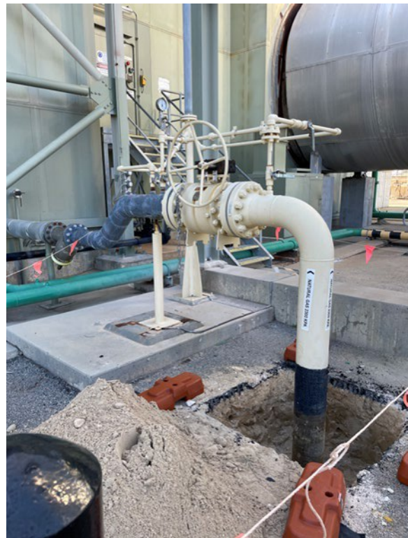
Figure 1.1: Example of unpiggable pipe
