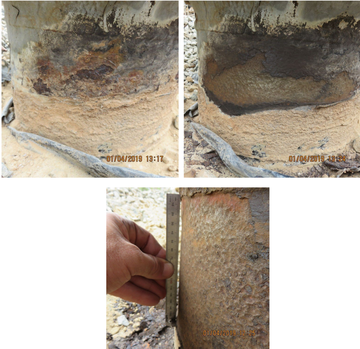
Figure 1.3: Photos of interface corrosion detected at facilities – features hidden behind the tape wraps
