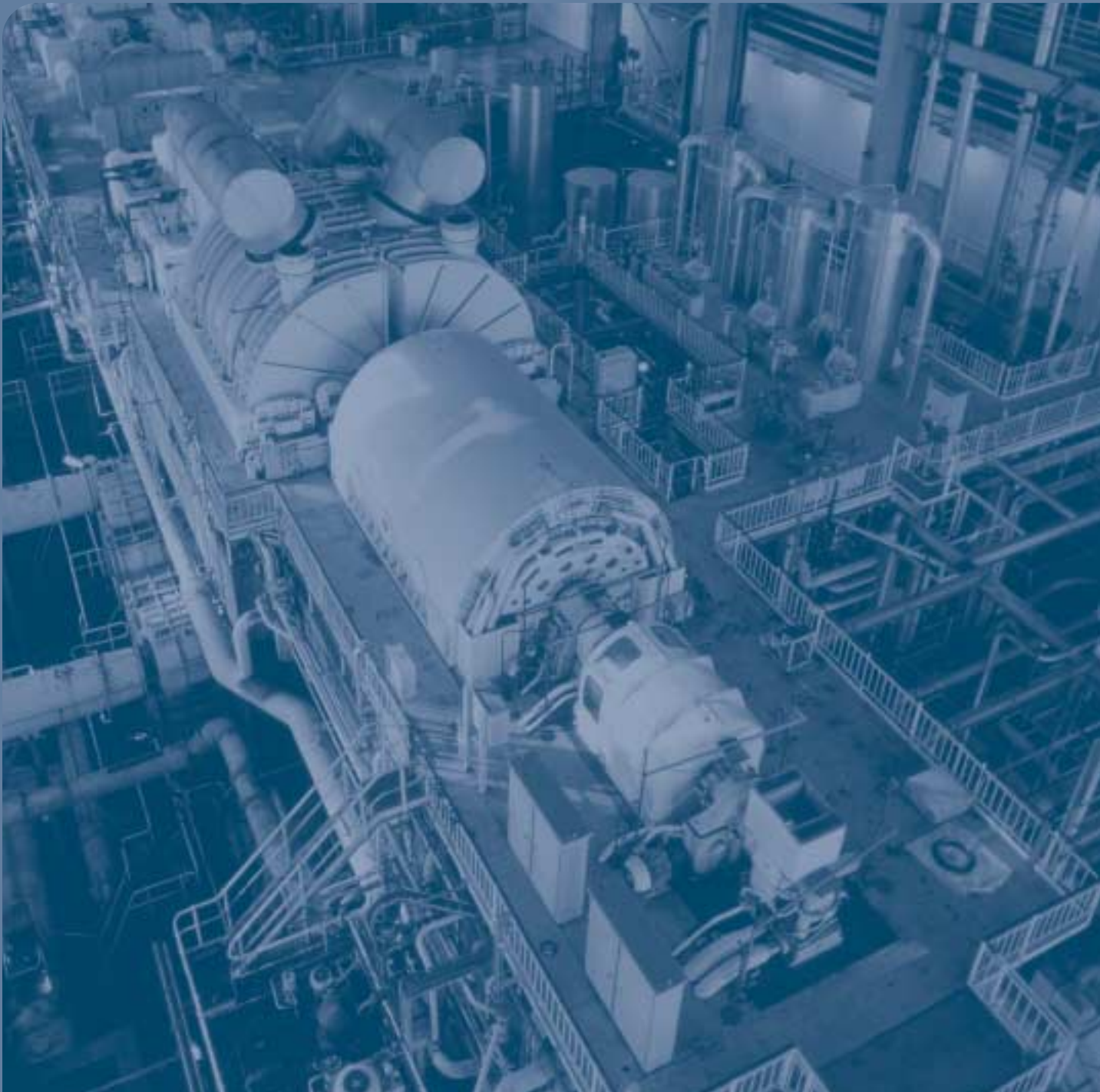
Turbine hall at Kwinana Power Station - a major gas user
