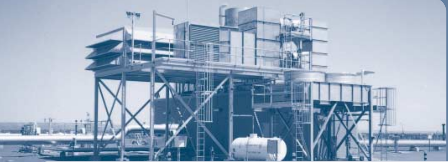
Compressor Station on the DBNGP
