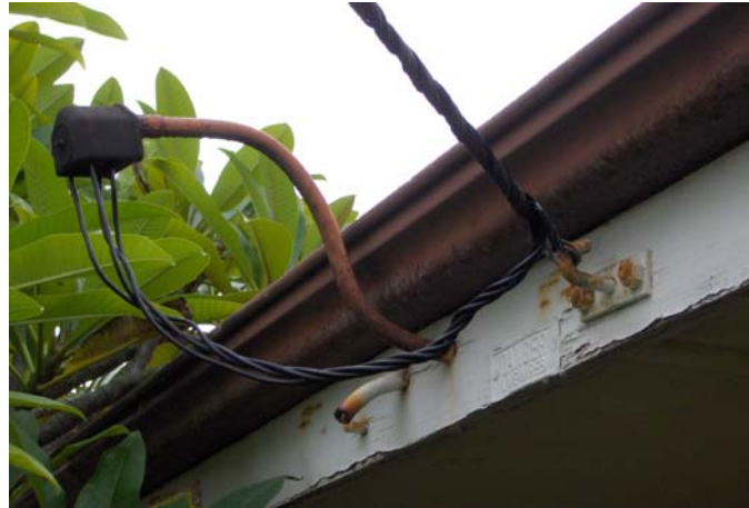
Figure 7: Example of a goose neck termination and preformed steel termination. The insulation on the wires entering the goose neck may be abraded, resulting in the goose neck becoming live. Under certain conditions the roof can also become live and hence be a further hazard.
