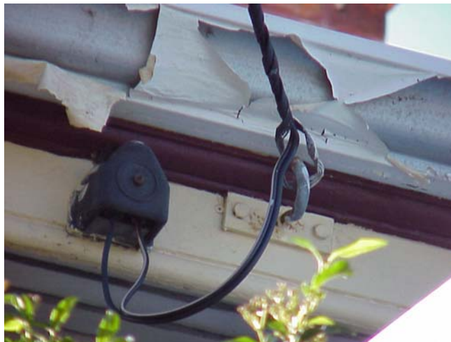
Figure 4 Example of a compromised service. The helical clamp is directly connected to the supporting bracket and, being too close to the metal roof, can make this live when wet and become a hazard
